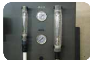
Concentrated and permeate flow meters.
