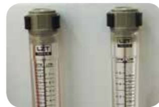
Flow meters reading of concentrated and permeate.
