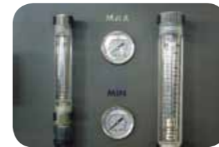
Concentrated and permeate flow meters
