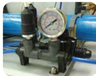
High and low pressure switches and pressure gauge.
