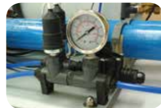
High and low pressure switches and pressure gauge.
